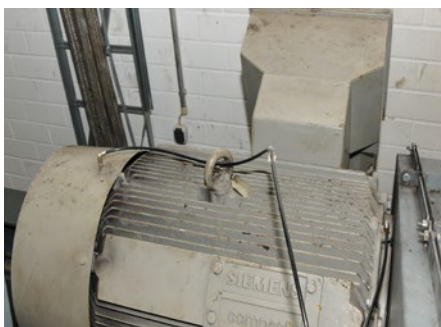
Lubricant supply on the fan drive
